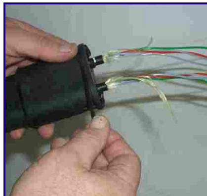
41 Wrap the strip of mastic around the cablegrip under upper lip to create a type of "O" ring.
