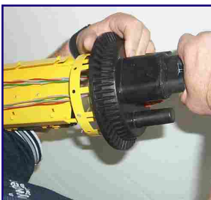
43 Pull rubber cablegrip and the cables through until the lower lip extrudes from the port ( DO NOT PULL ON BASKET ).
