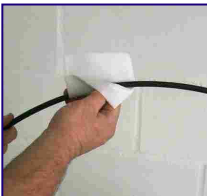
7 Clean the cable for a length of 4 metres for looped cables and 2 metres for single cable applications.
