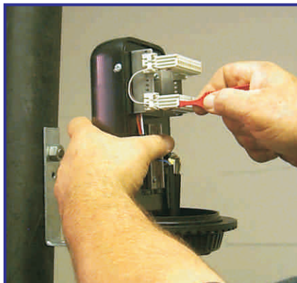
32 Connection between the exchange lines and the local lines are made with jumper wires.
