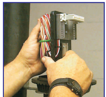
27 Carefully and neatly coil and fold cable pairs behind the Jointing Compartment support frame.
